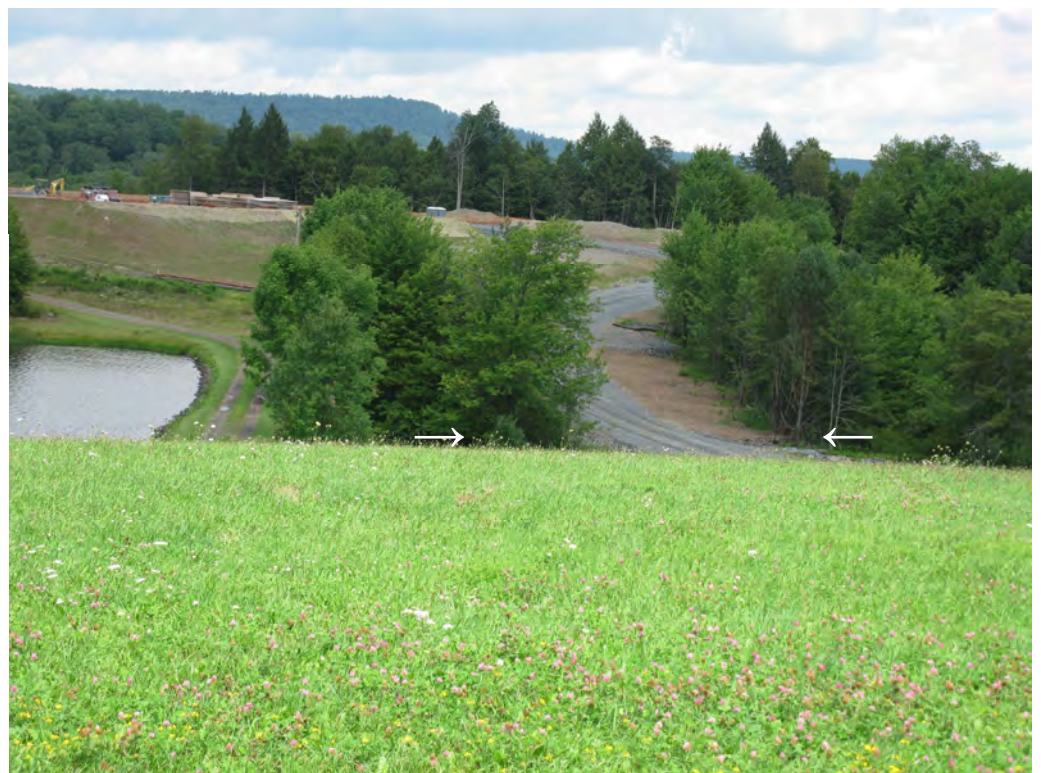
PHOTO F: View northward of the access road toward the Benspond Wellpad. The road was constructed across an EV stream (unnamed tributary to Elk Creek, at white arrows), and the riparian forest was cleared, without any PADEP Chapter 105 permit, because the drainage area here is less than 100 acres, and so the crossing was “waived”.
