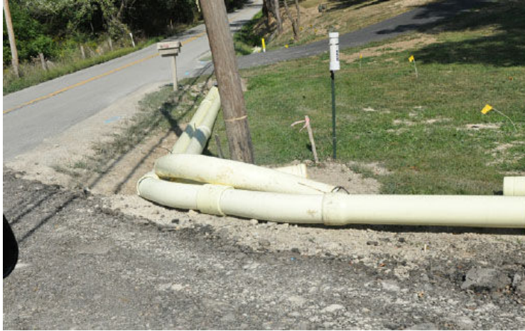
Gas well water lines clog road drainage culverts in Washington County PA.
